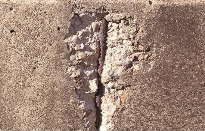
Figure 2-2 Corrosion and spalling induced by carbonation.
