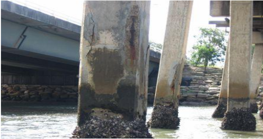
Cracked concrete bridge structures (SOURCE: RTA)
