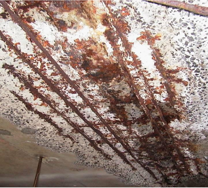
Figure 2-1 Corrosion of steel reinforcement in concrete structures
